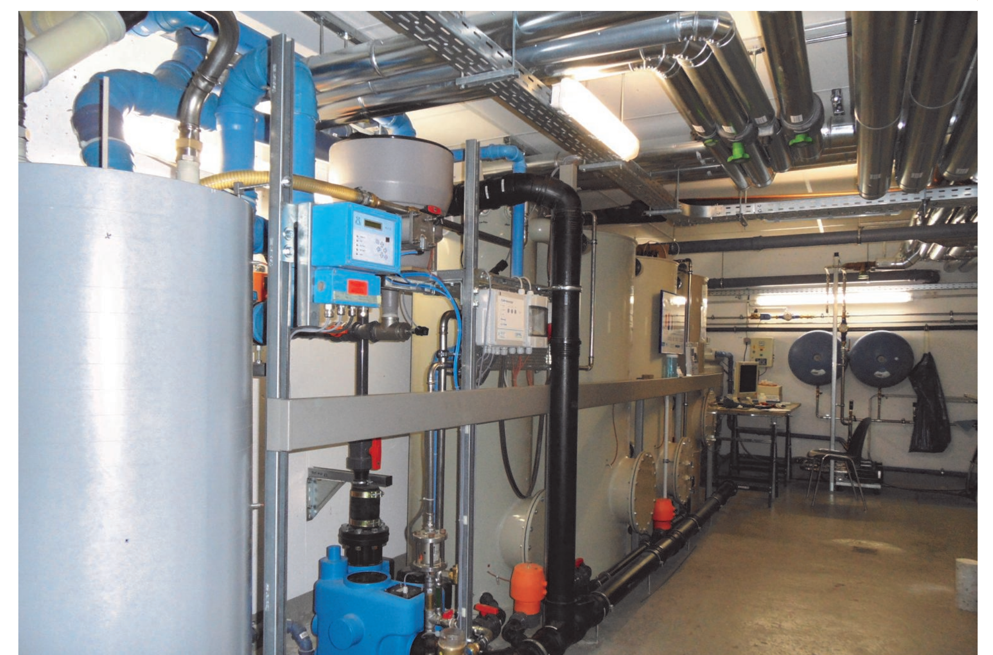
Photo 2: Greywater recycling combined with heat recovery. The combined system is placed in the basement where the building's heating system is also found, occupying an area of 9 m 2 (approx. 0.1 m 2 /person).
